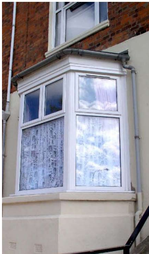
Unauthorised and insensitive replacement uPVC windows and doors result in the loss of much of the architectural character of a property.
