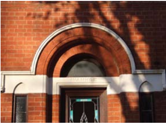
A detail of the side elevation to 2 Shaftesbury Avenue showing the Romanesque style arch above the front door.
