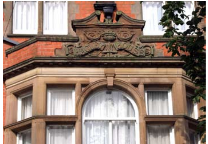
At 24 St. James Road the elaborate stone carved broken top pediment was designed to impress visitors.
