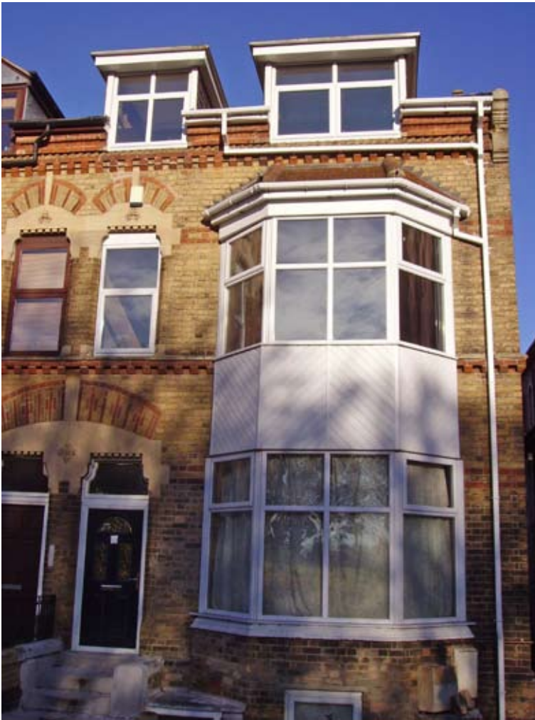
Insensitive replacement with uPVC windows, doors, fascias and rainwater goods, has resulted in the loss of much of the architectural character of this property.
