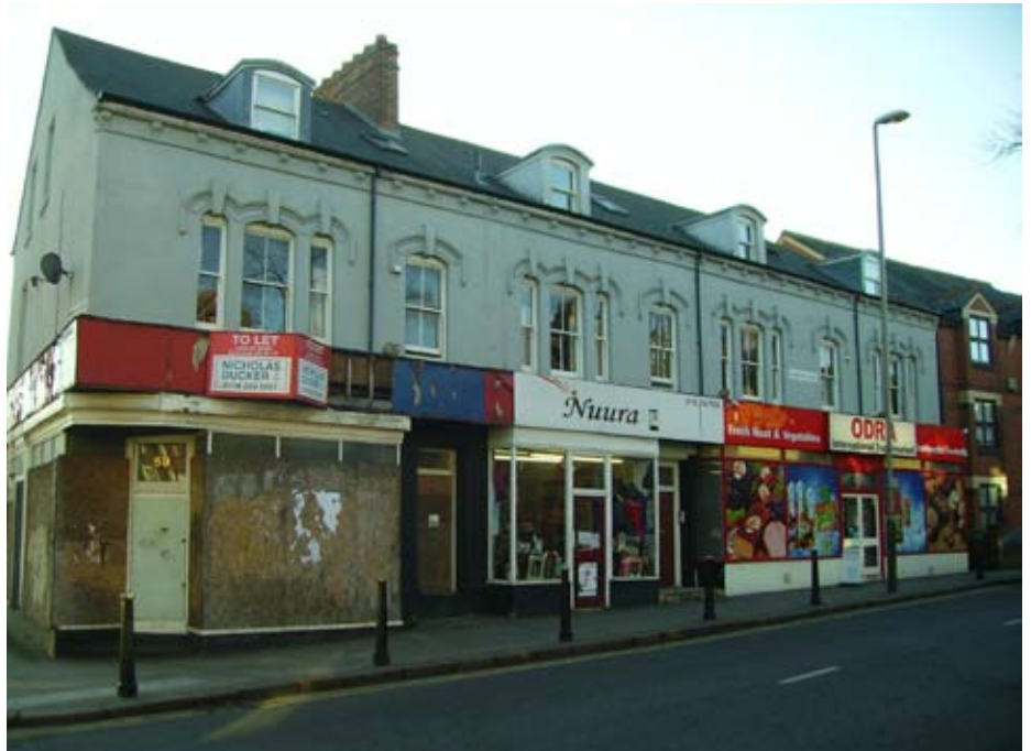
Numbers 55-59 Evington Road was originally a single retail showroom and has since been subdivided into three small shops. The signage and shopfronts are of poor design and lack any sense of coordination.
