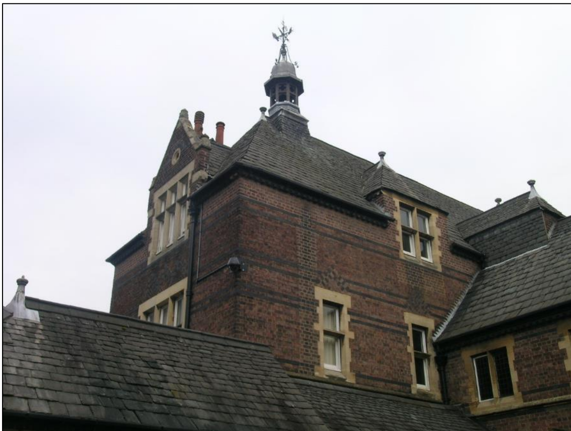
Figure 43: Westcotes House, with its elaborate elevations with blue brick and sandstone dressing, and complex roofscape, topped with a lead clad turret with a weathervane.
