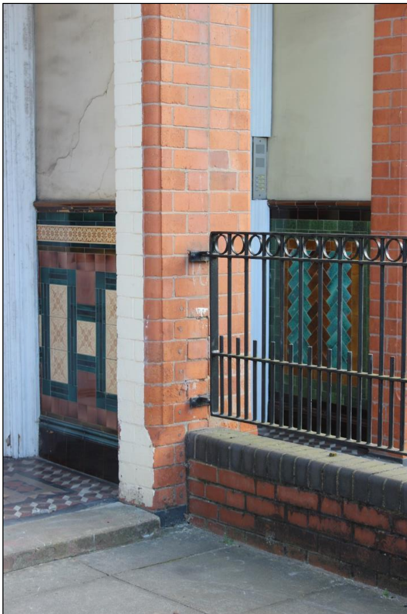
Figure 37: The intricate original tiled decoration on the inside faces of the porches at 46-48 Fosse Road South.
