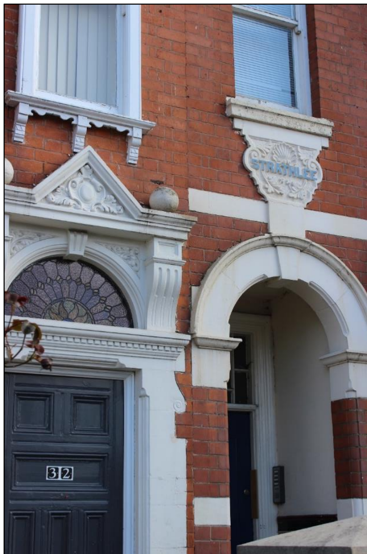
Figure 52: The carved stone and timber architraves, arches, brackets, pediments and name plaques at 32-34 Fosse Road South, original to these properties.
