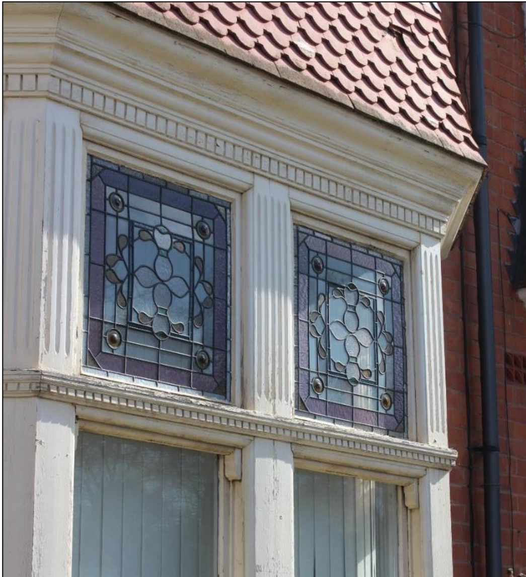
Figure 58: The stained-glass leaded windows at 30 Fosse Road South, set in intricately moulded joinery.
