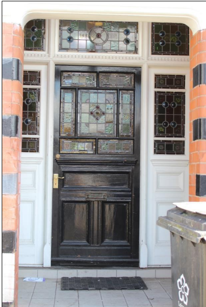
Figure 60: The original doorway with glazed timber panels at Cromford House, 20 Fosse Road South.
