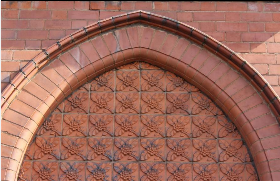
Figure 48: The red brick pointed archway to the side elevation of the Former Primitive Methodist Chapel, with moulded clay tiling to top.
