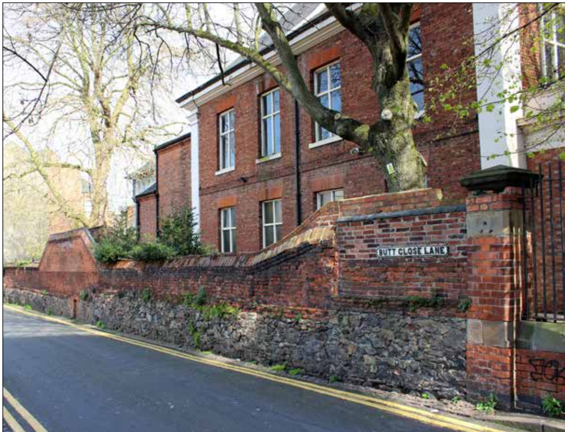
The boundary wall on Butt Close Lane is made of a of stones and bricks of varied styles and likely dates from the 18th Century.
