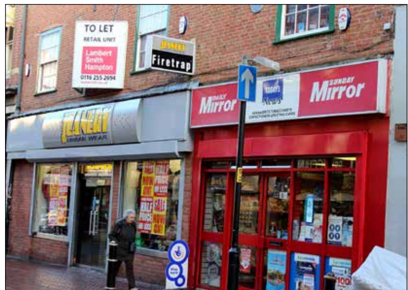
The shopfronts at 9-11 Church Gate don't relate well to the main building to the detriment of the building as a whole.
