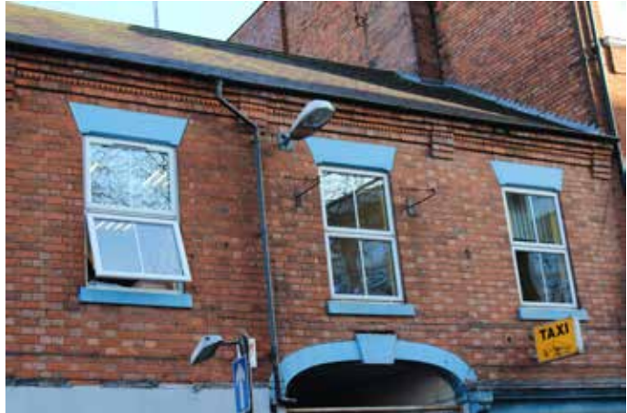
Inappropriate UPVC windows at 79 Church Gate
