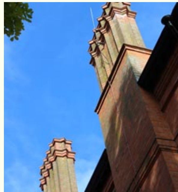
These impressive brick chimney stacks with moulded brick cornices can be found in Salisbury Road.
