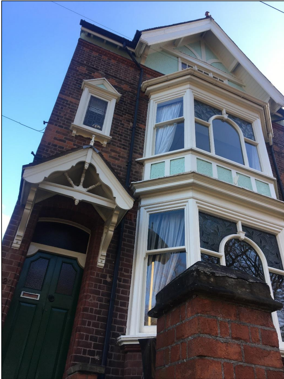
Figure 34: The original joinery at number 320 Fosse Road North is a rare and complete insight into the historic features that once decorated the frontage of a number of Victorian and Edwardian properties in the area.
