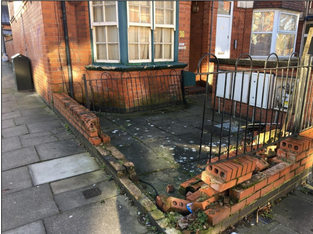
Figure 37: The damaged front brick wall at the corner of Henton Road and Glenfield Road.
