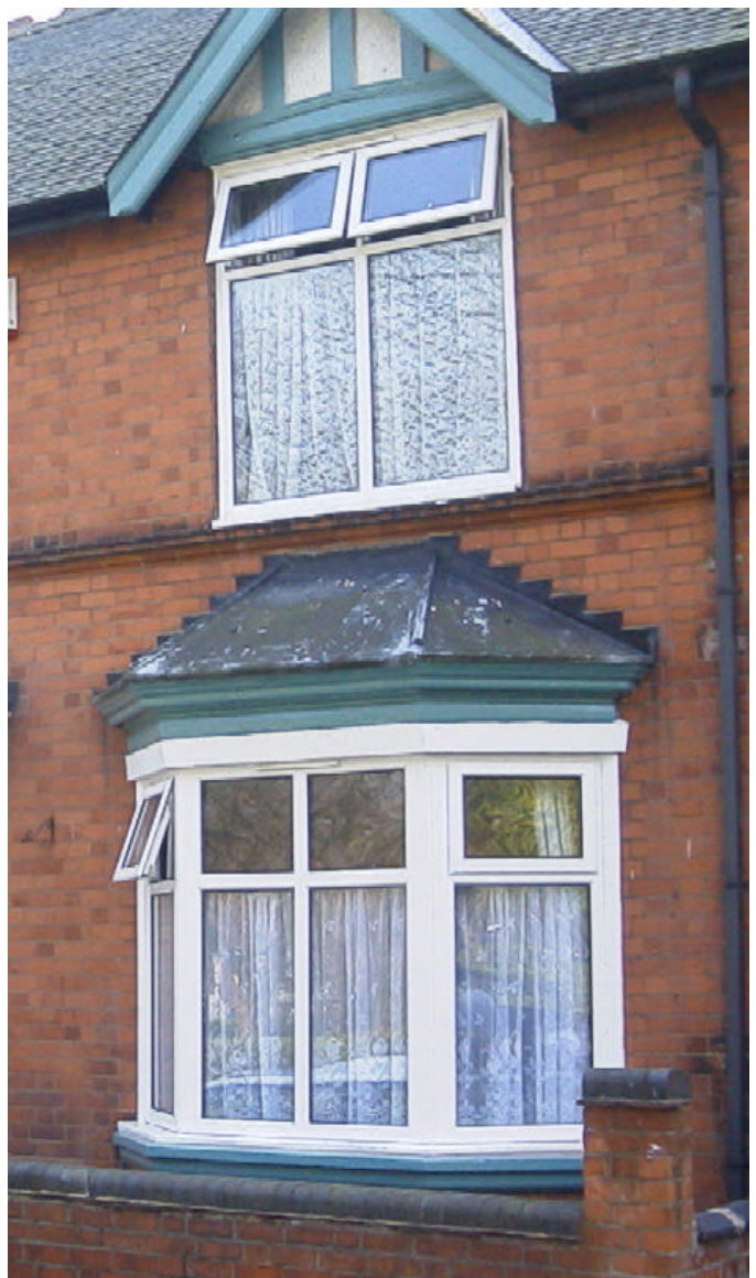
Unauthorised and insensitive replacement uPVC windows resulting in the loss of much of the architectural character of this property.
