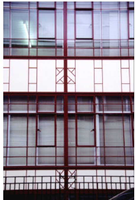
Nelson Street - The sophisticated art-deco style Crittall walling to the former Goddard's Plate and Powder premises, built 1934/5.
