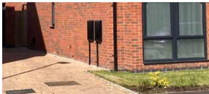
Figure 127. Utility Metres on the Side of Dwellings
