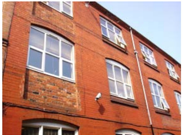
The insensitive replacement of original features such as windows and doors using an alien uPVC material, as shown here in Marble Street, can reduce the value of a building both visually, historically and financially.
