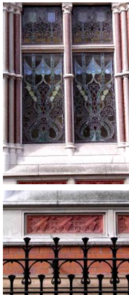
The City Council has a duty to preserve and enhance the character of conservation areas, to ensure that distinctive architectural qualities (as here at 31 Granby Street) are maintained for future generations.
