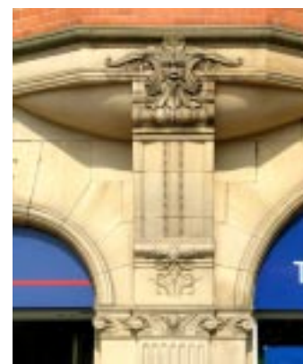
Carved stone detailing to the preserved façade of the former Royal Hotel, Horsefair Street.
