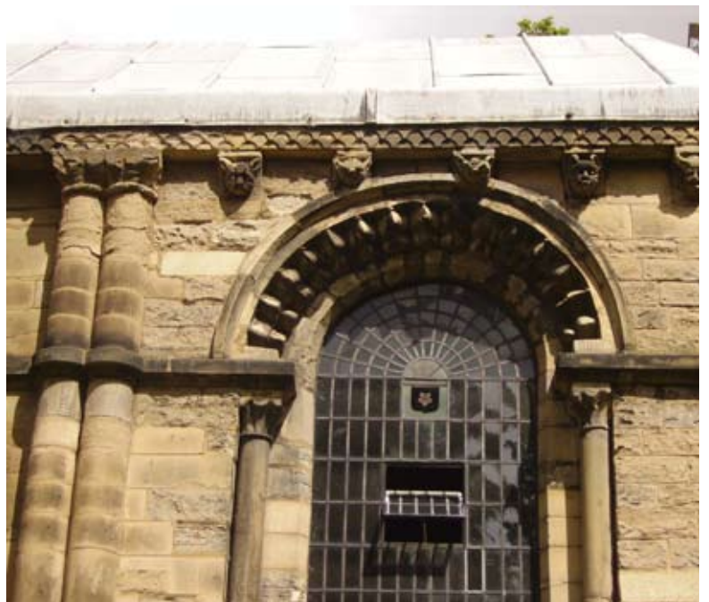
St. Mary de Castro; one of the Norman semi-circular arched windows to the south elevation.
