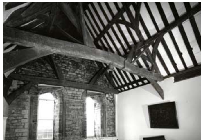
Part of the Castle Hall interior showing some of the original 12th century timbered roof structure.
