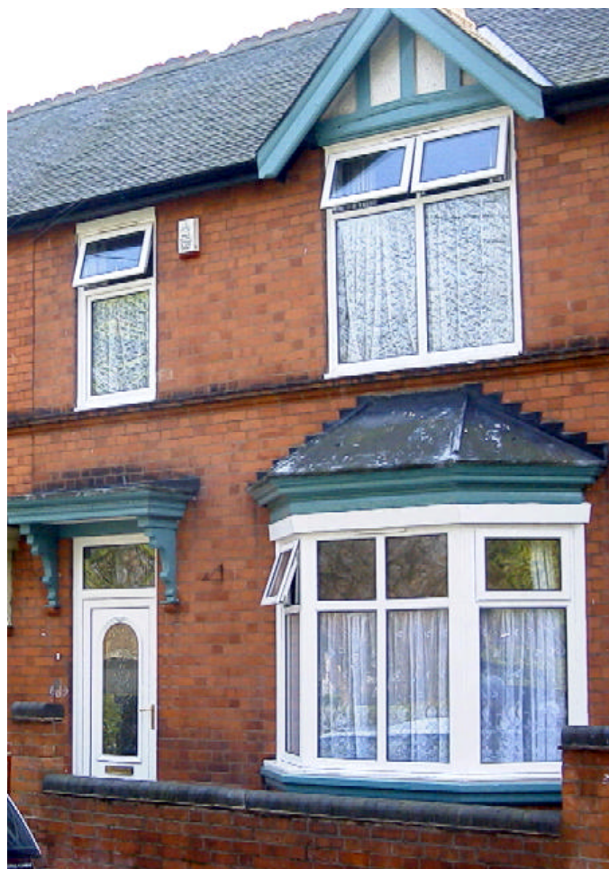
Unauthorised and insensitive replacement uPVC windows and front door resulting in the loss of much of the architectural character of this property.
