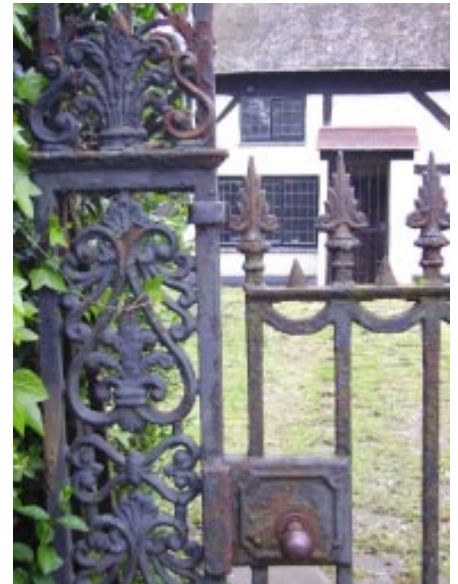
Detail of anthemion and palmette ironwork decoration to the gatepier at 106 Tennis Court Drive.
