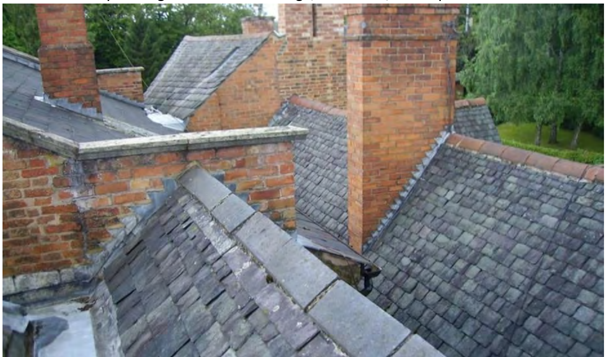
The varied and expansive historic roofscape of Knighton Hall, clad with Swithland slate with lead flashing.
