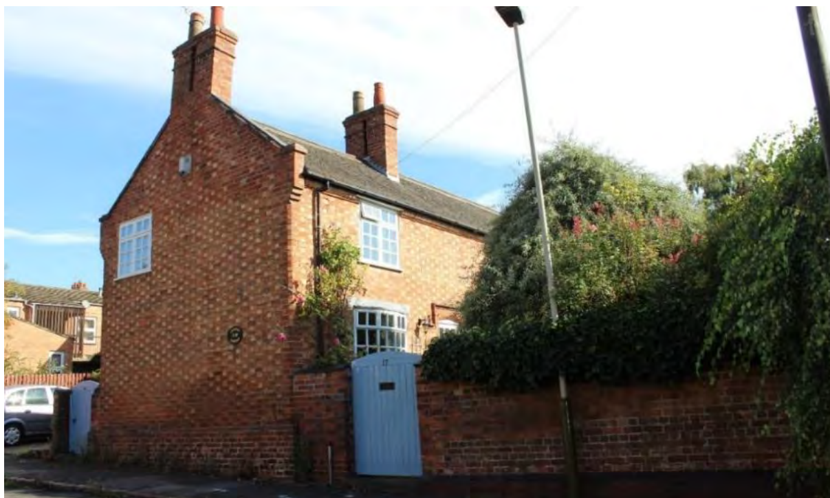
Gilliver Cottage: chequered brickwork in Flemish bond, animates the otherwise 'blank' gable
