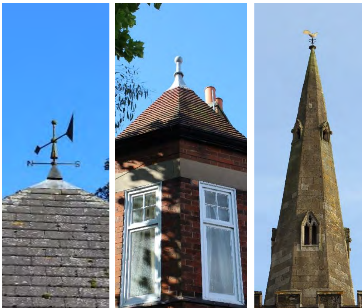
The rooftop features at Attenborough Arboretum Information centre (left), Gardiner House (centre) and most notably to St Mary Magdalen's Church animate the local skyline.
