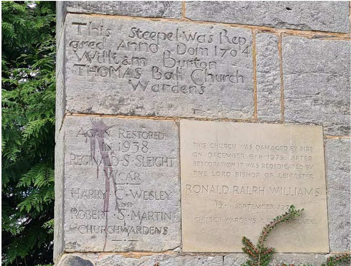
Details of the ashlar in buttress to the south west corner of the church tower. The inscriptions record repairs to the tower in 1704 and 1938 and the restoration of the whole church following a fire in 1975
