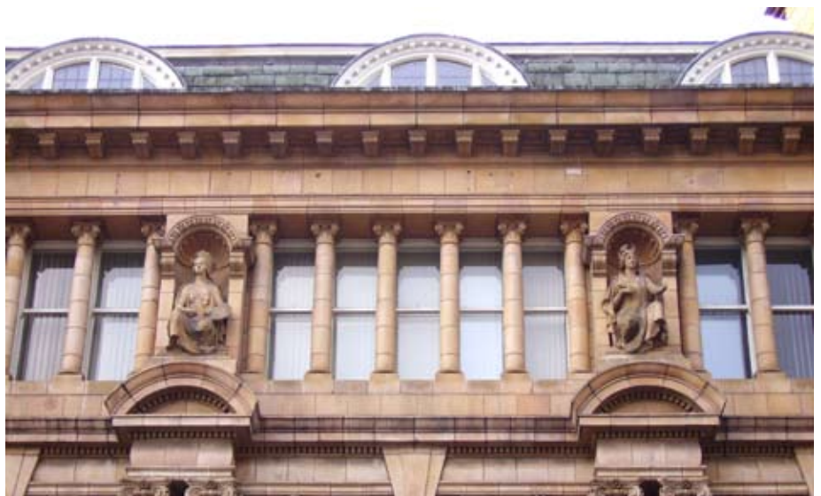
Part of the former General Newsroom designed by Joseph Goddard and dating from 1898. This replaced William Flint's building of 1838, (see page 28).
