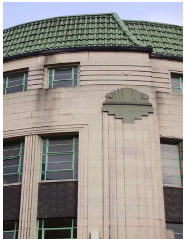
Green glazed tiles, Portland stonework, bronze panels and steel window frames are used to great effect at 128 - 132 Granby Street.
